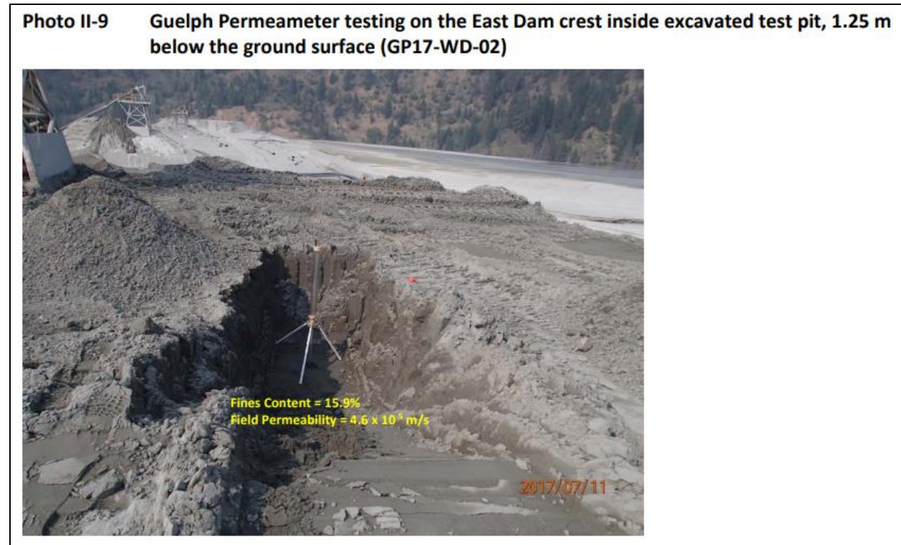
Figure 20c. Guelph permeameters are used to measure the in-situ saturated hydraulic conductivity of the uncompacted cycloned sands that are used to raise the tailings dams. The as-built reports by AMEC (2016a) and Klohn Crippen Berger (2017b, 2018, 2019) document extensive testing of construction material. However, as the above photo of a Guelph permeameter in a test pit at a depth of 1.25 meters indicates, this testing has been carried out only on the material (uncompacted cycloned sand) that had been used to raise the tailings dams since the previous annual report. By contrast, there is essentially no documentation of any testing that occurred prior to 2015. Tetra Tech (2022) described the construction material for the starter dams (constructed in 1971) as “random” and stated that “there is limited data on the compacted cycloned sands that were used to construct the dam shell prior to 1980.” In fact, prior to 2015, it does not appear that construction was even carried out in accordance with the design. According to Tetra Tech (2022), “The reactivation design also called for a rockfill zone at the toe of the dams, extending back to the pre-2011 dam slope and 40 to 50 m above the dam toe. However, there is no indication that this was ever built; based on as-built records (KCB 2021b) [Klohn Crippen Berger (2021) in this report], the zone where rockfill was proposed to be used was constructed of cyclone sand ... The reactivation design also called for slope drains, similar in design to the 2014 crest drain (AMEC 2011), to be laid along the downstream slopes of the dams, but there is no evidence that these were installed.” Based on the contrast between the current quality of testing and the pre-2015 testing, as well as the extensive construction that occurred prior to 2015, the category for Level of Engineering in the area of Design – Testing was chosen as Average to Above Average (see Table 1b). Photo from Klohn Crippen Berger (2018).
