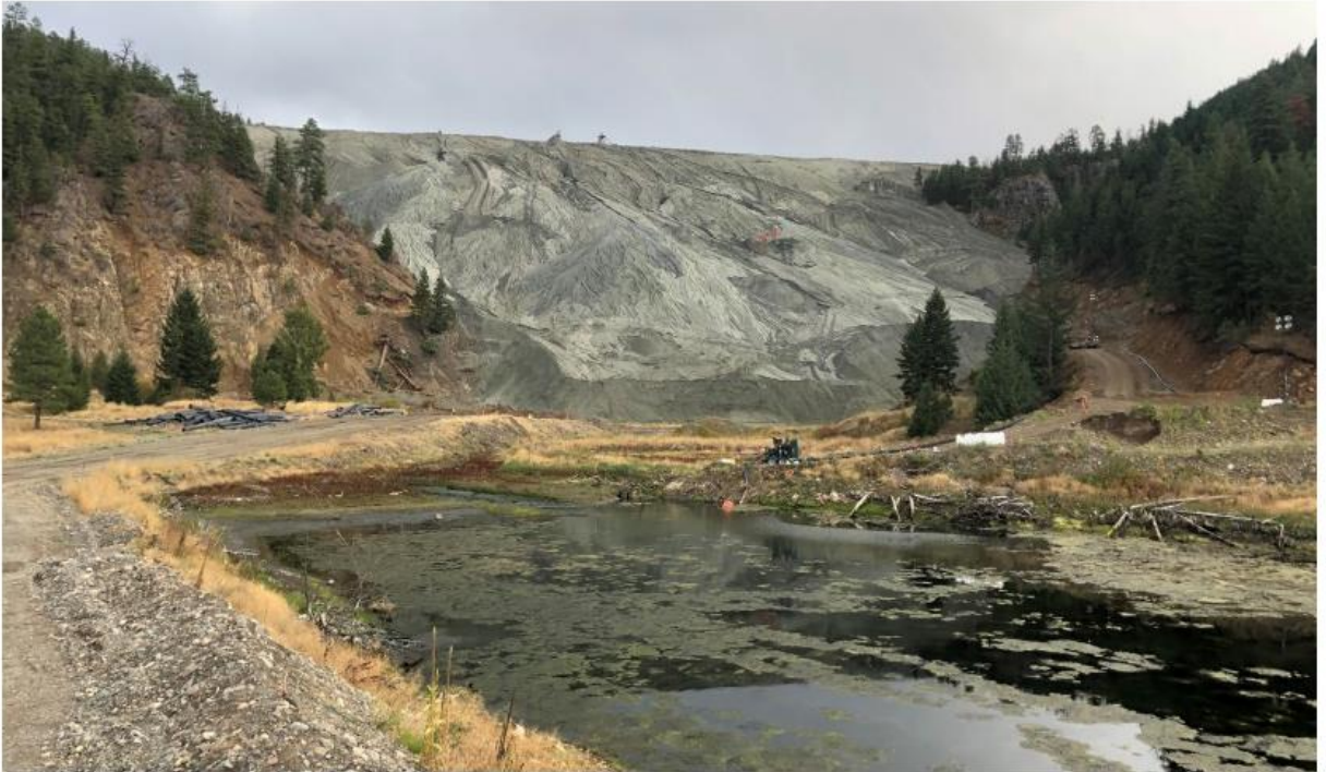
Figure 3b. At the end of 2022, the crest of the West Dam will be 973 meters above sea level, corresponding to an approximate height of 164.5 meters. The permitted crest elevation of 997 meters above sea level (corresponding to an approximate height of 188.5 meters) will be achieved in 2027. Photo from Klohn Crippen Berger (2021).
