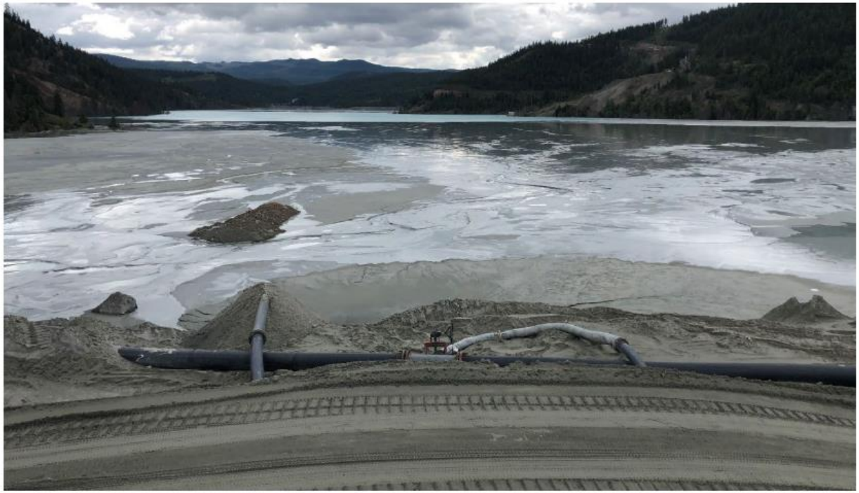
Figure 17a. The overflow from the cyclones (see Fig. 16) consisting of finer tailings and water is discharged from the crest of the West Dam toward the interior of the tailings management facility. The coarser fraction of the overflow settles closer to the dam crest to form a tailings beach (foreground of photo; compare with Figs. 2 and 11). The finest fraction of the overflow (slimes) is carried to the interior of the tailings management facility (background of photo; compare with Figs. 2 and 11). Photo from Tetra Tech (2022).
